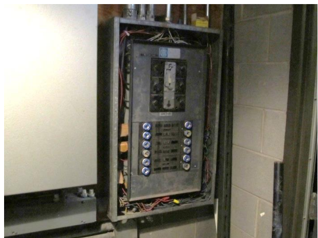
Fuse type circuit protection panel
