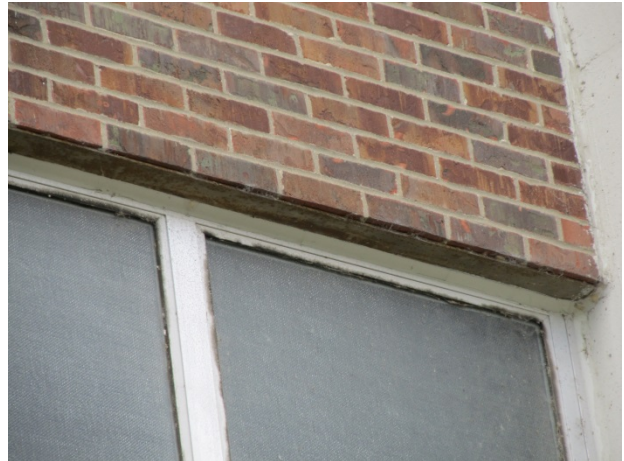
Rust at shelf angle and lack of flashing
