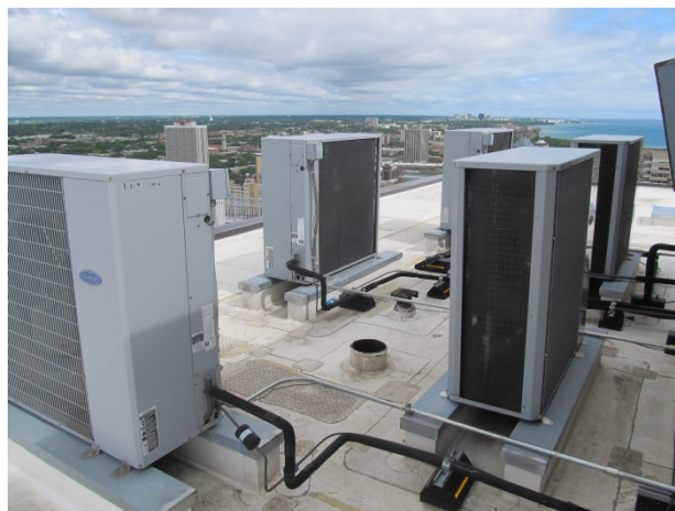
Condensing units for exercise and party room
