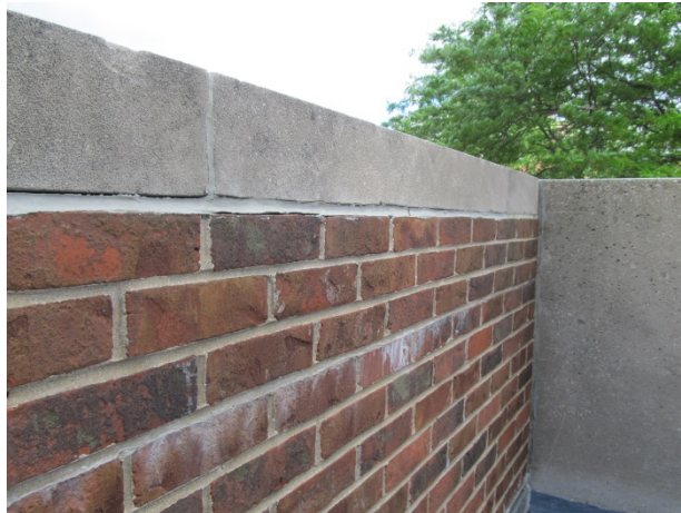
Lack of flashing beneath cap and efflorescence at base structure
