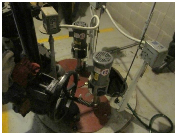
Sump/sewage ejection pumps
