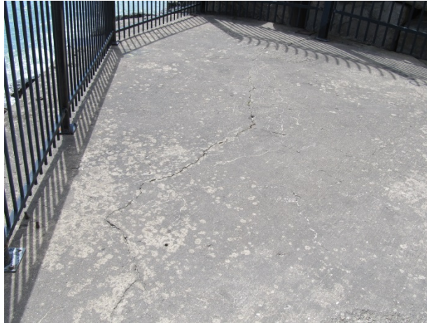
Fishing pier concrete cracks
