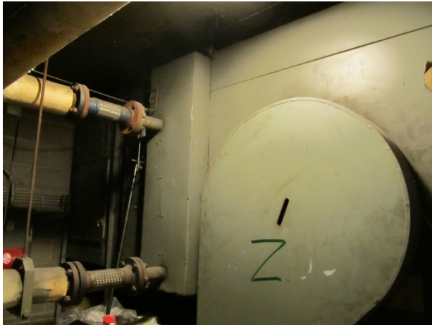
Corridor air handling unit
