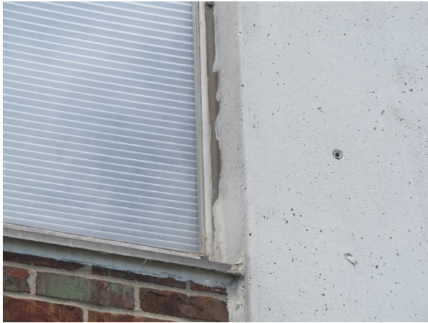
Varied sealant conditions at metal/concrete interface
