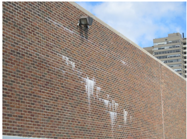
Efflorescence at base structure at east elevation
