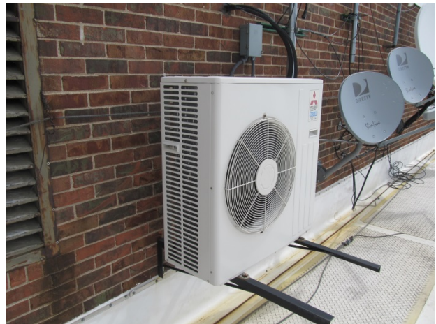
Condensing unit for elevator room
