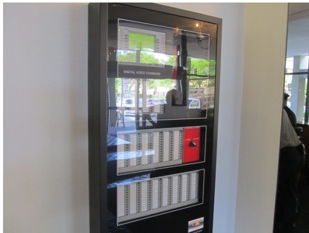
Central life safety panel
