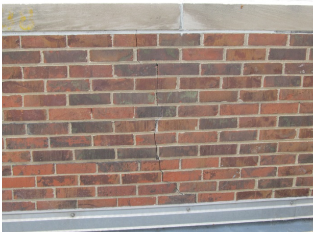
Crack in masonry at parapet wall at base structure
