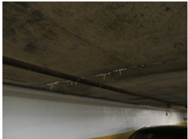
Evidence of water infiltration beneath west perimeter vaulted concrete
