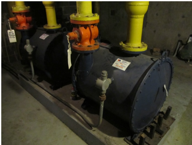
Gas booster pumps
