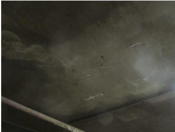
Evidence of water infiltration beneath 1st floor garage level
