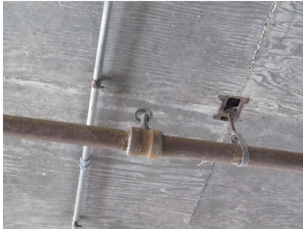
Fire sprinkler system head
