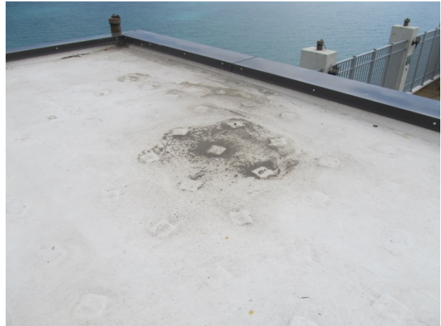
Evidence of lack of drainage at mechanical penthouse roof
