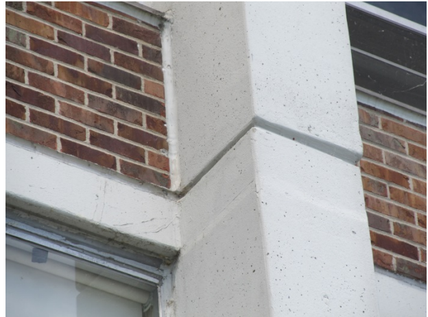
Sealant at brick/concrete interface
