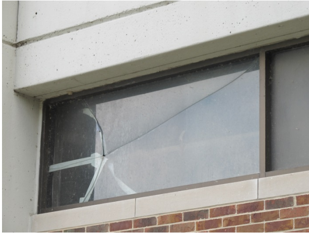
Cracked common window at garage
