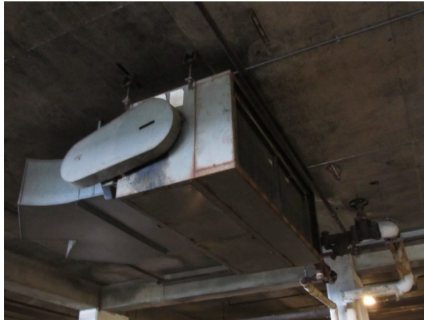
Garage unit heater
