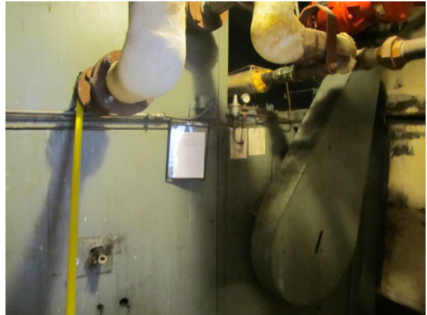
Air handling unit for 29 th floor
