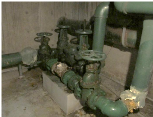
Valves at main water connection
