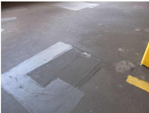
Numerous traffic coating repairs and areas of coating deterioration at 1 st floor
