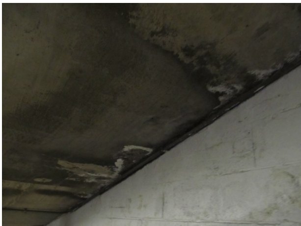
Evidence of water infiltration beneath 2 nd floor garage level
