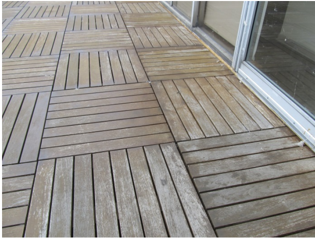
Sun deck wood finish deterioration
