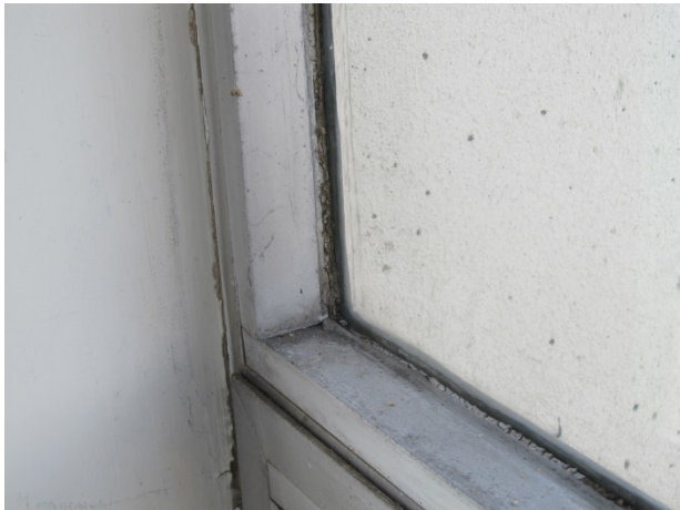
Seal failure at unit window
