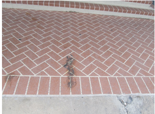
Concrete deterioration at lobby entrance area
