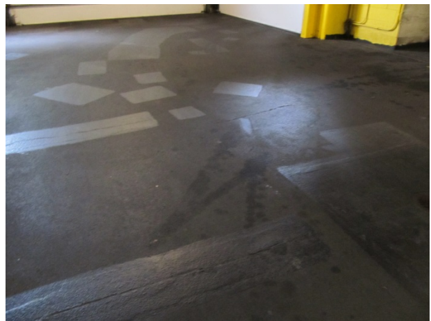
Numerous traffic coating repairs and areas of coating deterioration at 1 st floor
