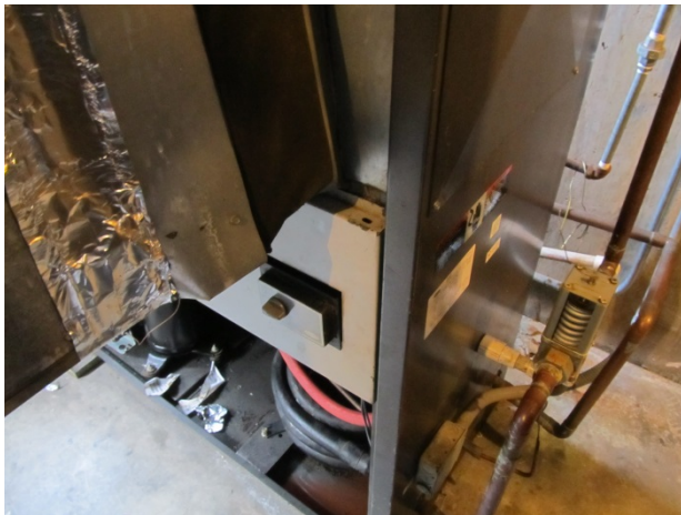
Air handling unit for 1 st floor
