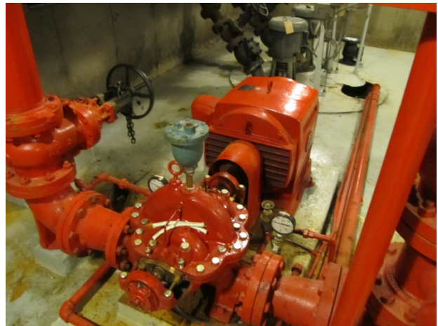
Fire suppression pump
