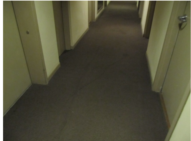
Stains at carpet
