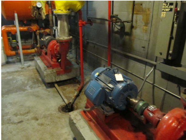
Building heating pumps
