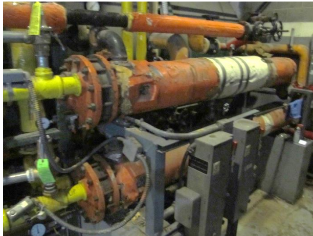
Domestic water heat exchangers
