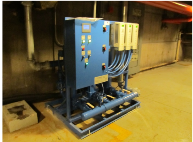
Domestic cold water pumps
