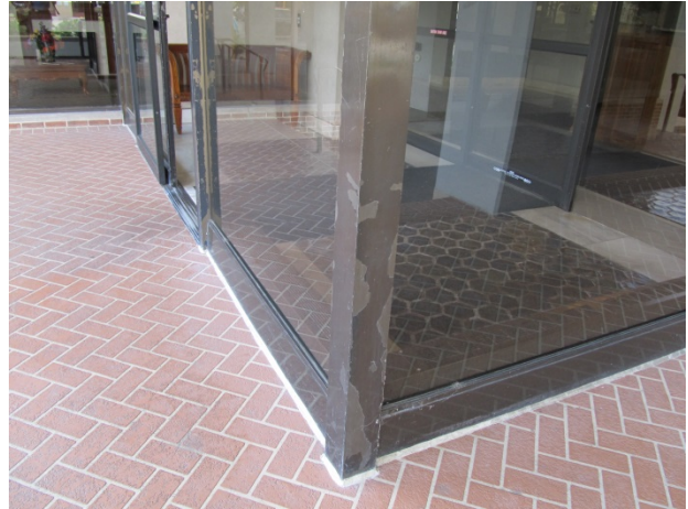
Finish deterioration at lobby window system
