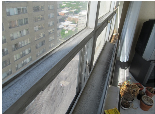
Lack of a gasket at hopper window
